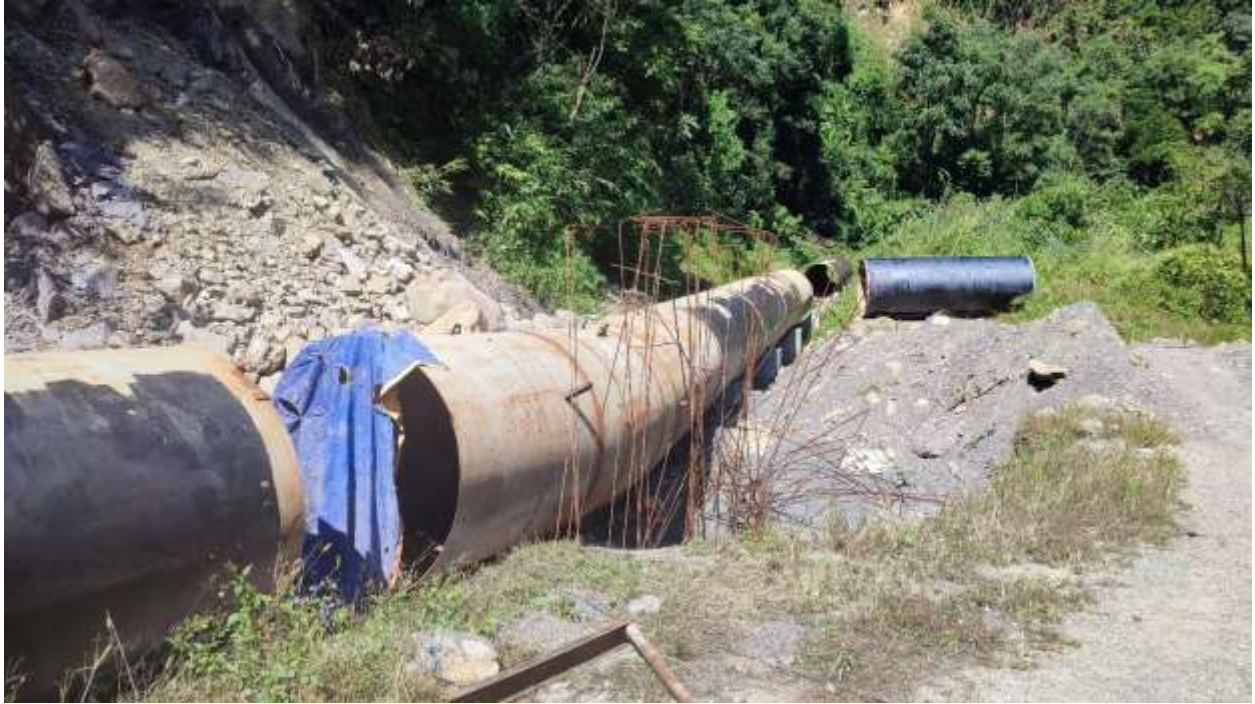
Landslide around AB6
