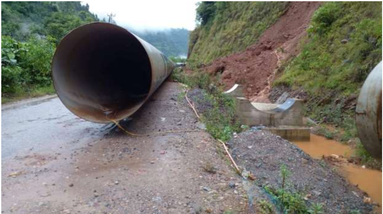
Landslide between IP42-IP44
