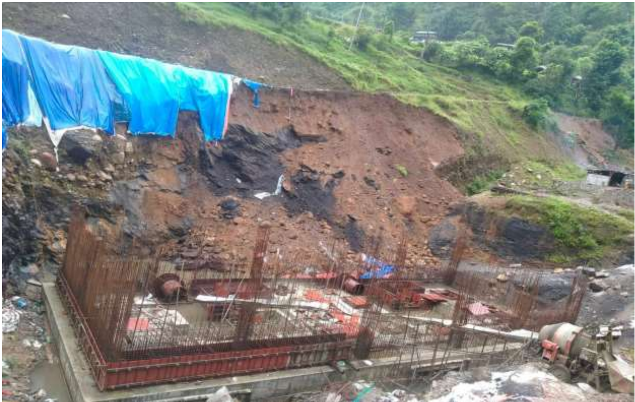
Landslide Behind Powerhouse
